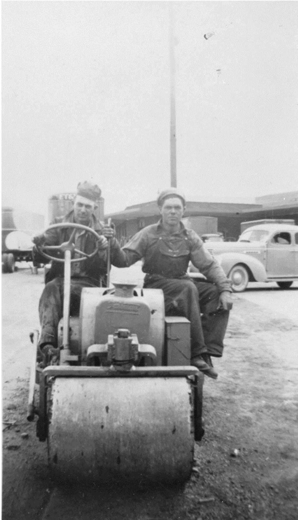
Figure 14. “Roller (front view) at Johnson City making repairs to Buffalo Street after 3 rd rail removal”. 43
