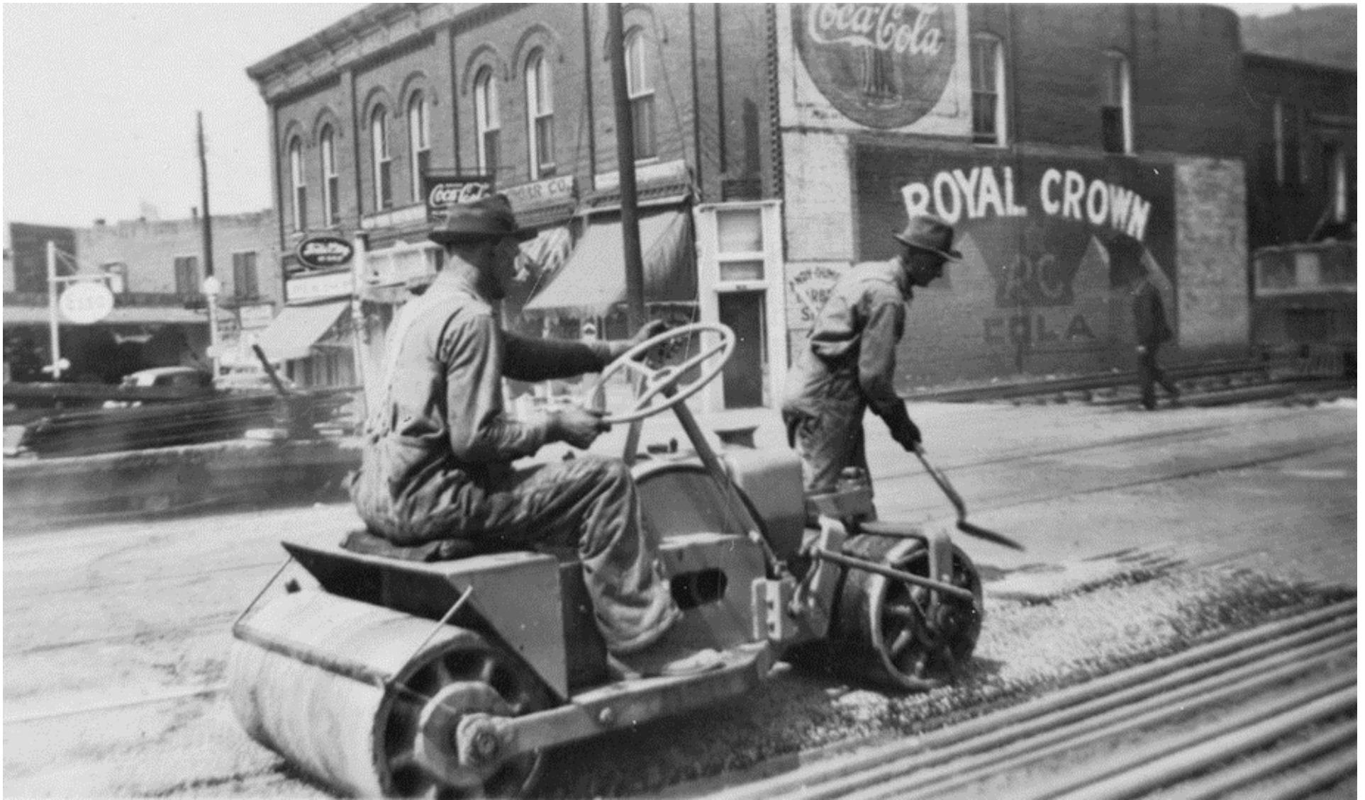
Figure 37. “Roller... at Johnson City making repairs to Buffalo Street after 3 rd rail removal” 147 “In September 1946, the third rail between Johnson City and Elizabethton was removed.” 148 Note the Coca-Cola and Royal Crown Cola signs on the south side of the Harr building, as well as the Esso sign in the left background. Also note that the cornice of the Harr building was intact when the third rail was removed.
