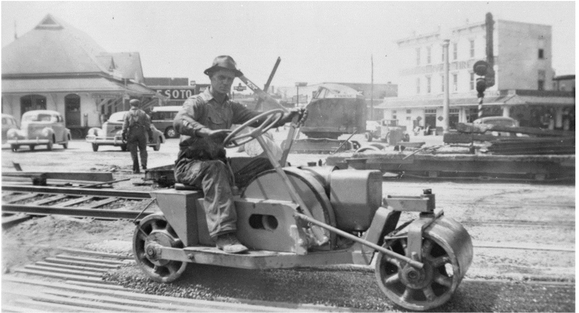
Figure 12. “Roller (side view), [E.T. & W.N.C.] digger in background at Johnson City, making street repairs after 3 rd rail removed,” 39 “In September 1946, the third rail between Johnson City and Elizabethton was removed.” 40 Also note the ET&WNC tracked shovel behind the roller, as well as the crossing signal and the Free Service Tire Company building on the right of this photograph.
