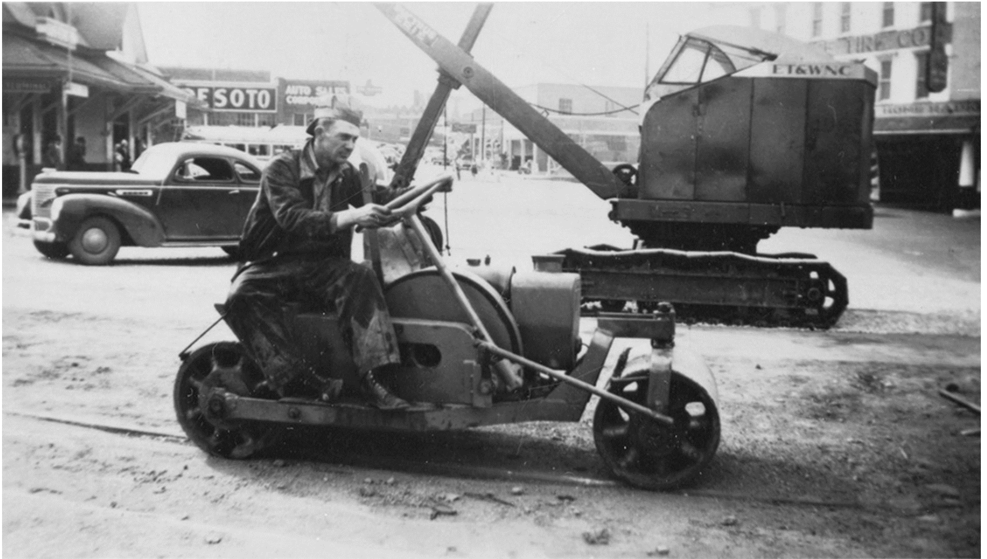
Figure 13. “Roller... at Johnson City – making street repairs to Buffalo Street after 3 rd rail removal”. 41 “In September 1946, the third rail between Johnson City and Elizabethton was removed.” 42 Also note the E.T. & W.N.C. “digger” behind the roller.
