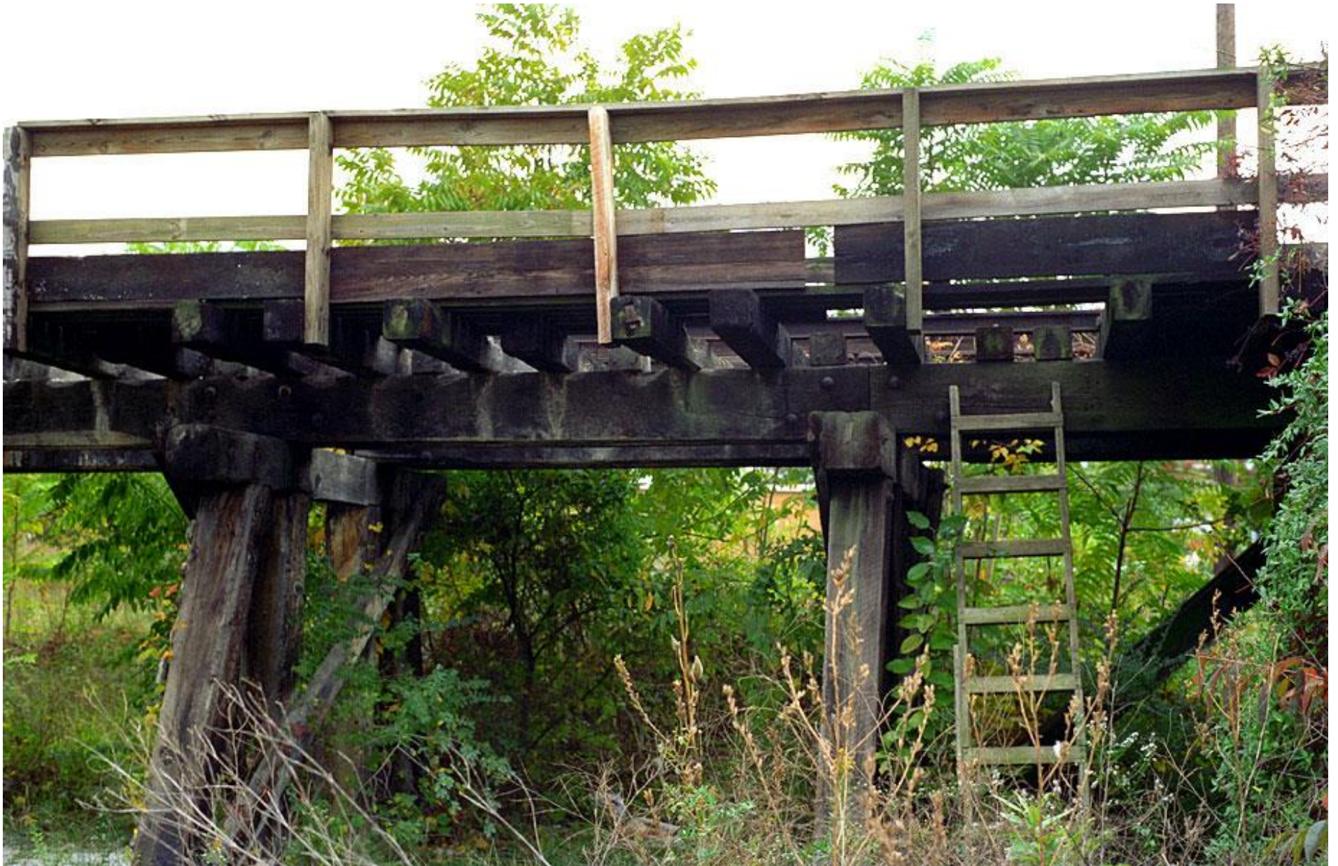
Figure 4. Chris Ford wrote: “October 1995... Coal Trestle in Johnson City” This is how a coal platform is built. This trestle is just east of Roan Street on Cherry Street in Johnson City. It's not technically a street in this section although you can drive on it. The massive legs are 12 x 12s. The stringers are 6 x 16s...” 20
