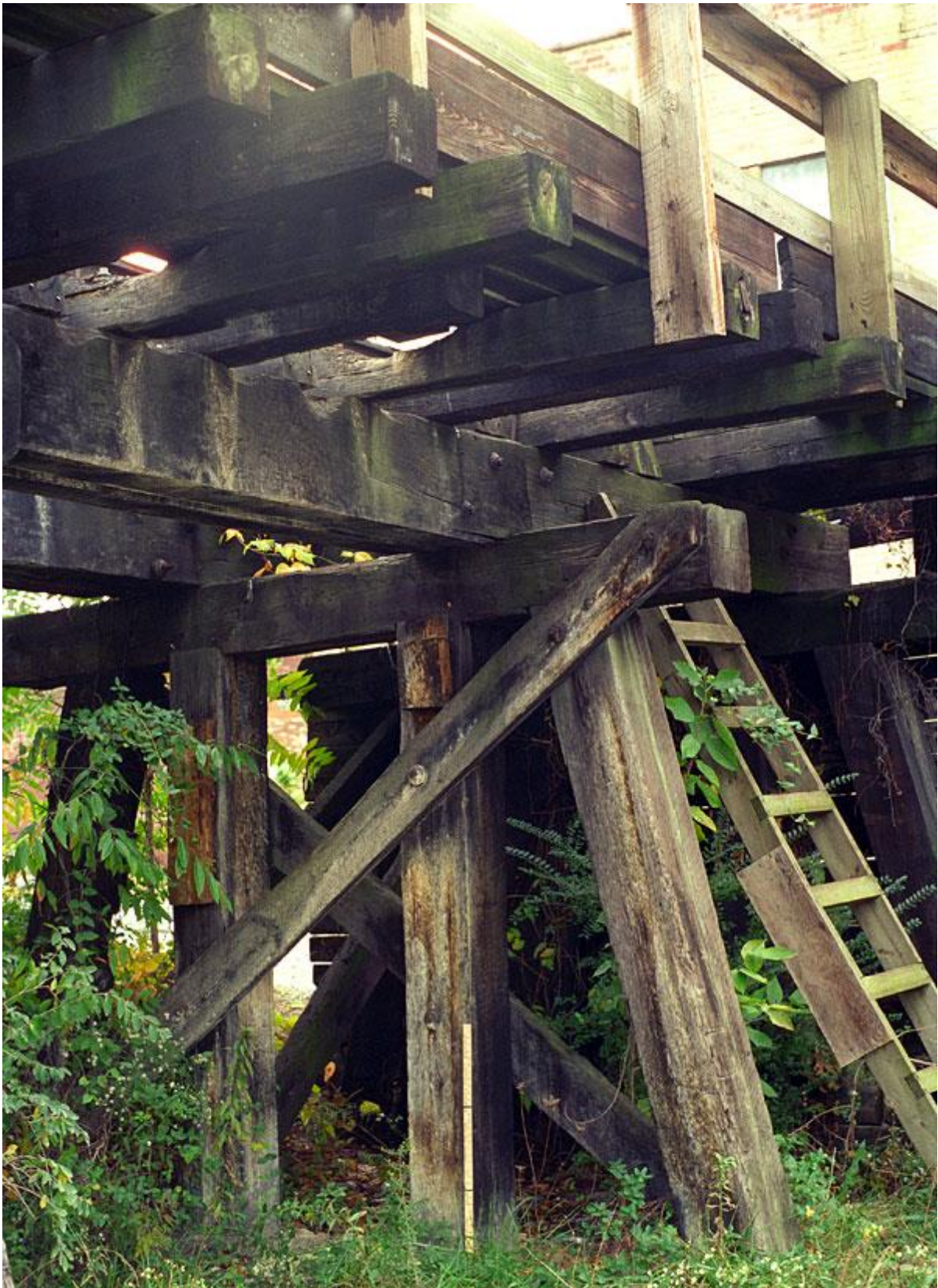
Figure 5. Chris Ford wrote: “This structure on Cherry Street is very similar construction to the historic ET&WNC coaling and transfer trestle in the Johnson City yard. The trestle in this photo was gone in 1999.” Note the building once occupied by the Johnson City Coal, Ice & Cream Company is in the top right of this image. 21
