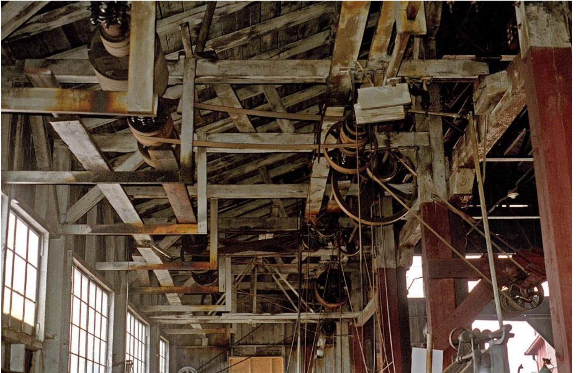
Figure 60. Chris Ford wrote of this photograph: “June 1991 – Johnson City Enginehouse Beltdrive Machinery – The still-in-place, and (I assume) still-working, leather belt pulley system was very impressive. This is at the back of the building. I’m guessing it has been there as long as the enginehouse.” 71
