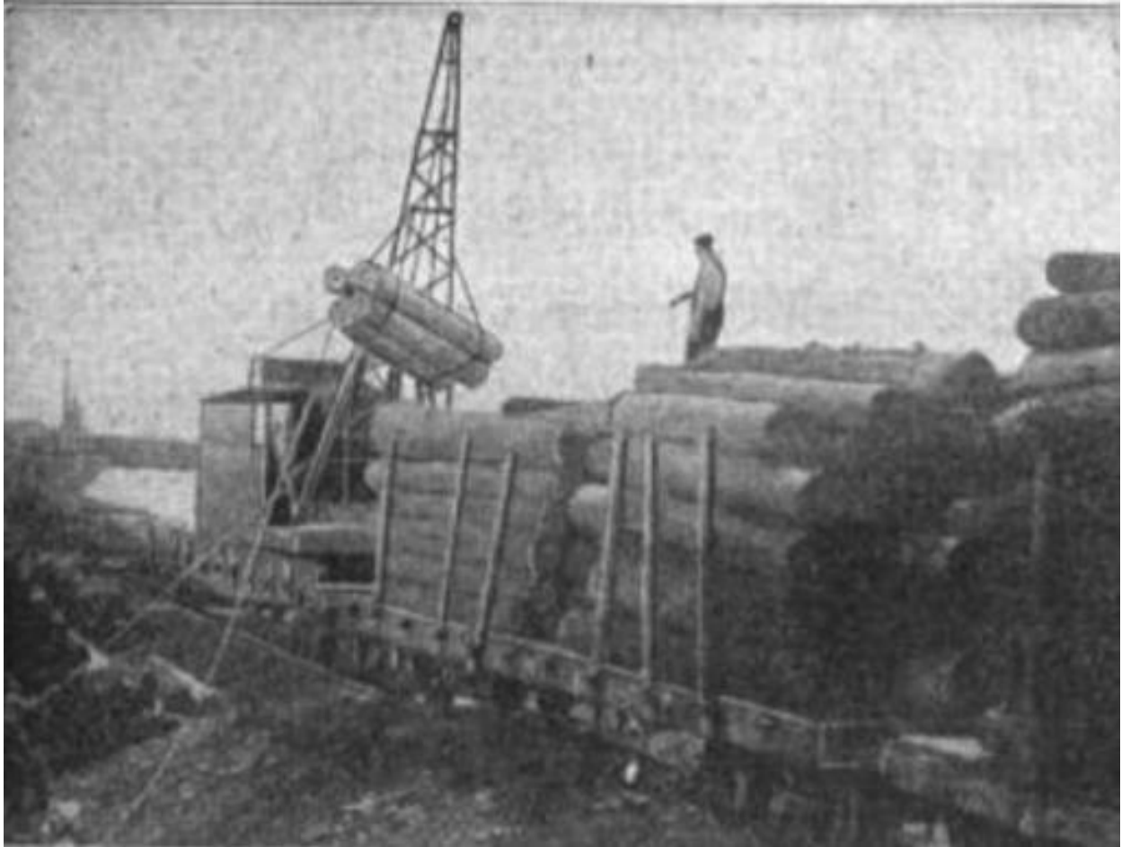
Figure D – 2. “L. Stephenson Co., Wells, Mich. Capacity 100,000,000 feet annually. All their loading is done with Raymond Gasoline Loaders, as shown. Cleveland Cliffs Iron Co., Marquette, Mich., are using nine Raymond Log Loaders. They are also heavy operators. Our Loaders are the most economical operated of any Loaders on the market.” 124
