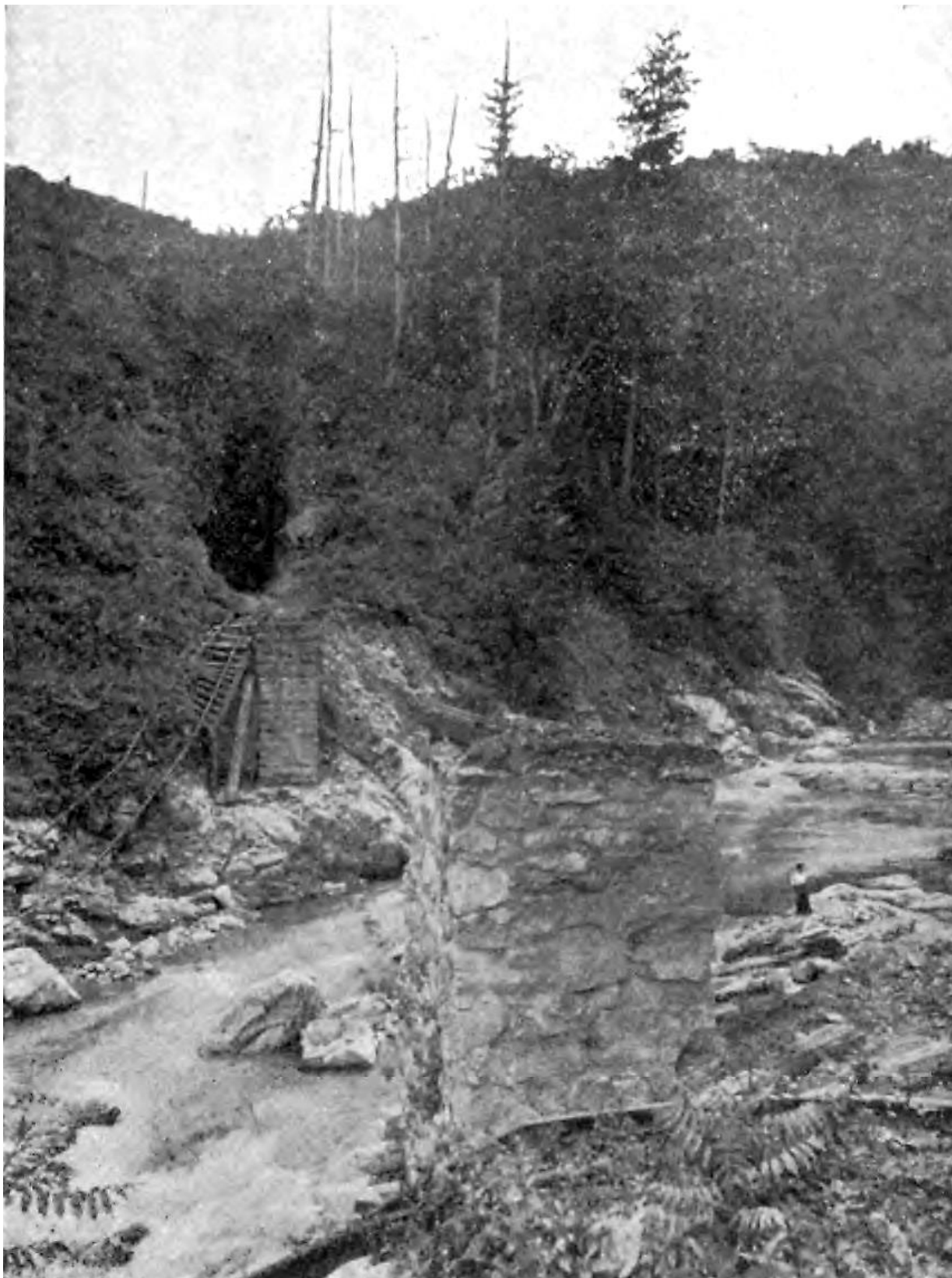
Figure 4. "Wreck of a Railroad Bridge, Doe River, Tenn.", after the flood of 21 May 1901. This appears to have been Bridge #6 of the E.T. & W.N.C., with the entrance to Tunnel #4 visible across the river. Although no mention has been found on the damage sustained by the Uptegrove operation at White Rock Mountain as a result of this flood, at a minimum, Uptegrove could not ship any lumber until after 23 July 1901. 24
