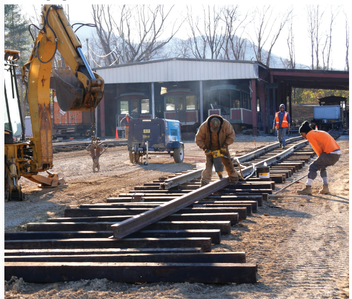
Narrow gauge track laying at Doe River Gorge - 2023. Photo courtesy Mark Milbourne.
